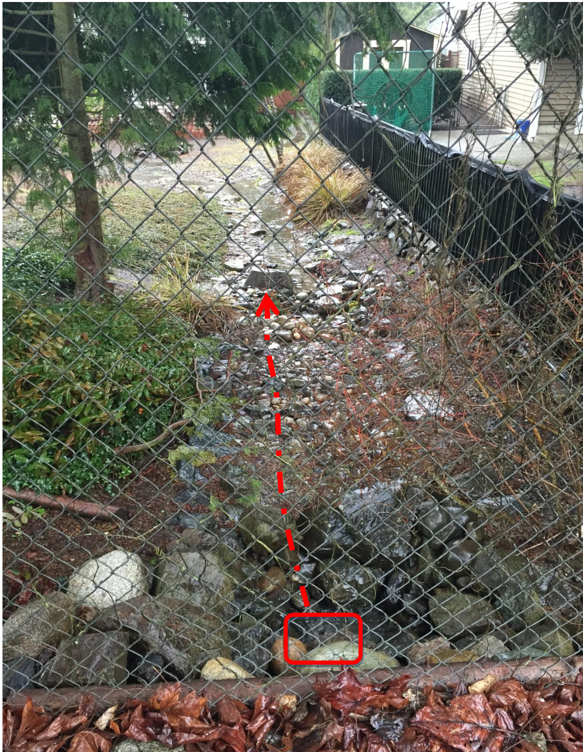
Photo 3 Current Site Condition (looking from the northeast corner of the site towards north existing discharge point)
