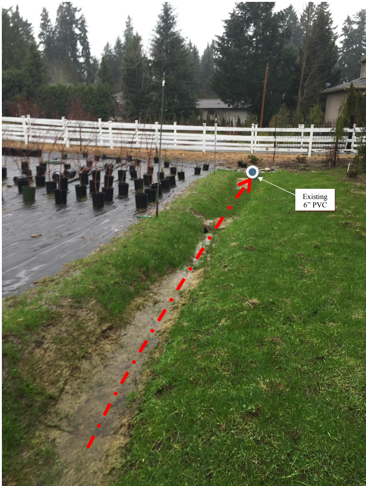
Photo 2 Current Site Condition (Existing ditch enters the 6" pipe and continues flowing toward northwest corner of the site, looking from the southeast corner of the site towards northwest corner)
